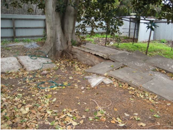
Concrete path damage from a Ficus root system
