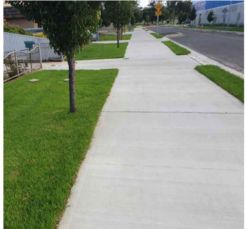
| New wider shared footpaths for safer walking and cycling and stormwater control
